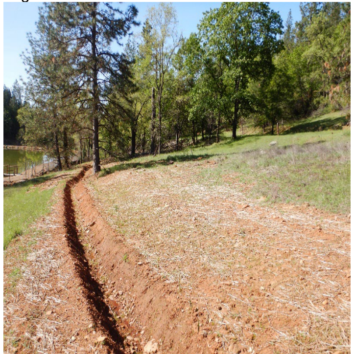
Photo No. 8: Tailwater collection ditch associated with the land application area.
