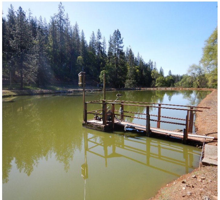
Photo No. 4: Wooden structure that supports pump for the spray aeration system and piping that leads to the land application area.
