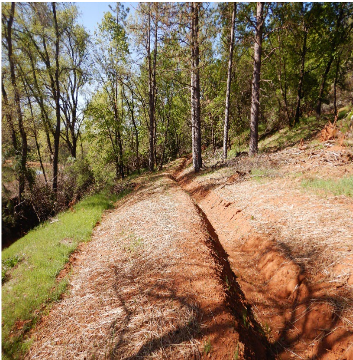
Photo No. 7: Tailwater collection ditch associated with the land application area.
