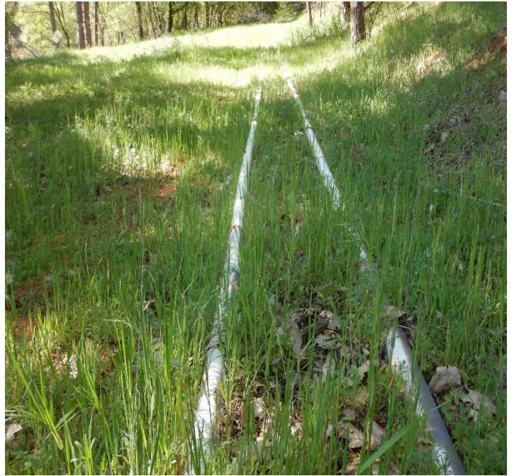
Photo No. 6: Looking south at the land application area and the PVC piping used for drip irrigation.
